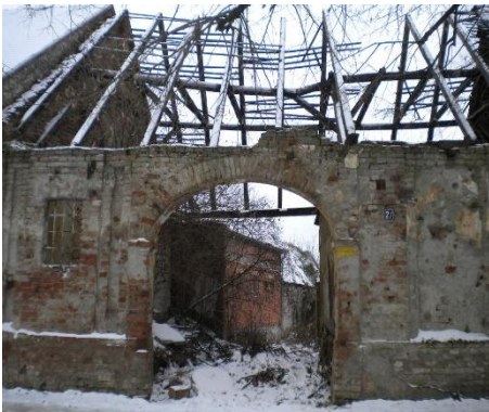
Home in Vukovar Croatia, destroyed in 1991 during the Croatian War of Independence (photo taken 2011)
